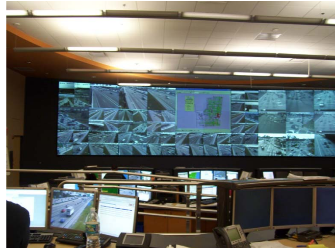
District 4 RTMC Video Wall
