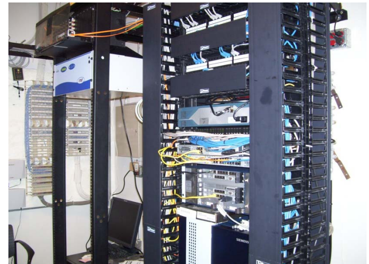
District 7 RTMC Equipment room
