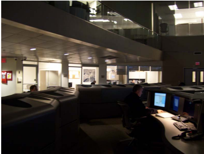
District 6 RTMC Floor
